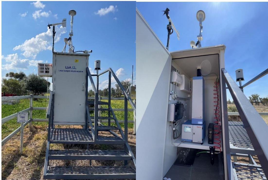
Figure 1: TEOM installed at Lanreef
